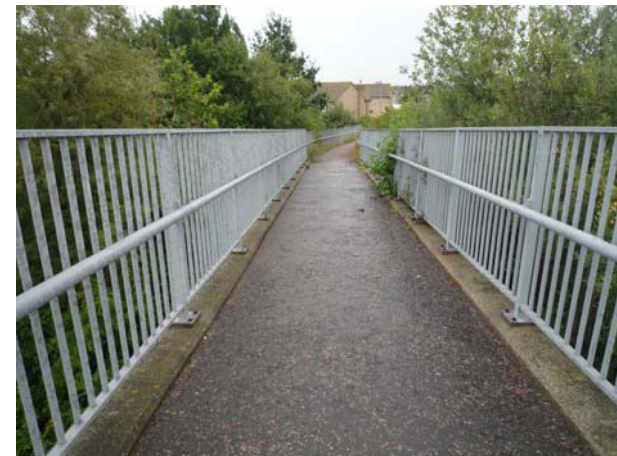
Handrails with poor colour contrast
