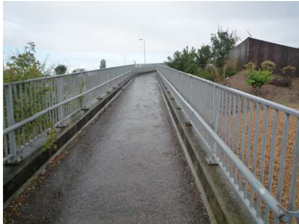
Poor colour contrasting handrails
