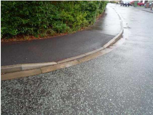
Dropped kerb with no blister warning
